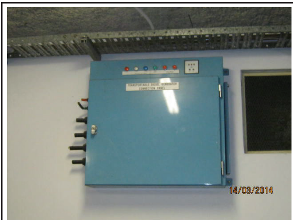
Photo 9: Disconnected power box to diesel AST
