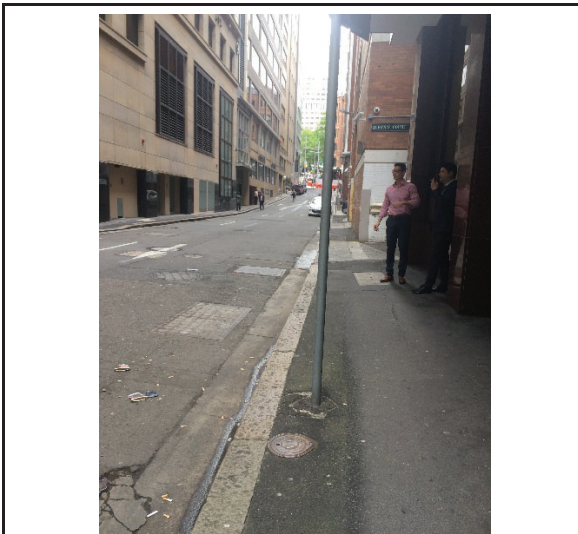
Photo 5: Potential dip/fill point on northern footpath of Dalley Street
