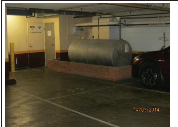
Photo 8: AST location on upper basement car park at 37 Pitt Street
